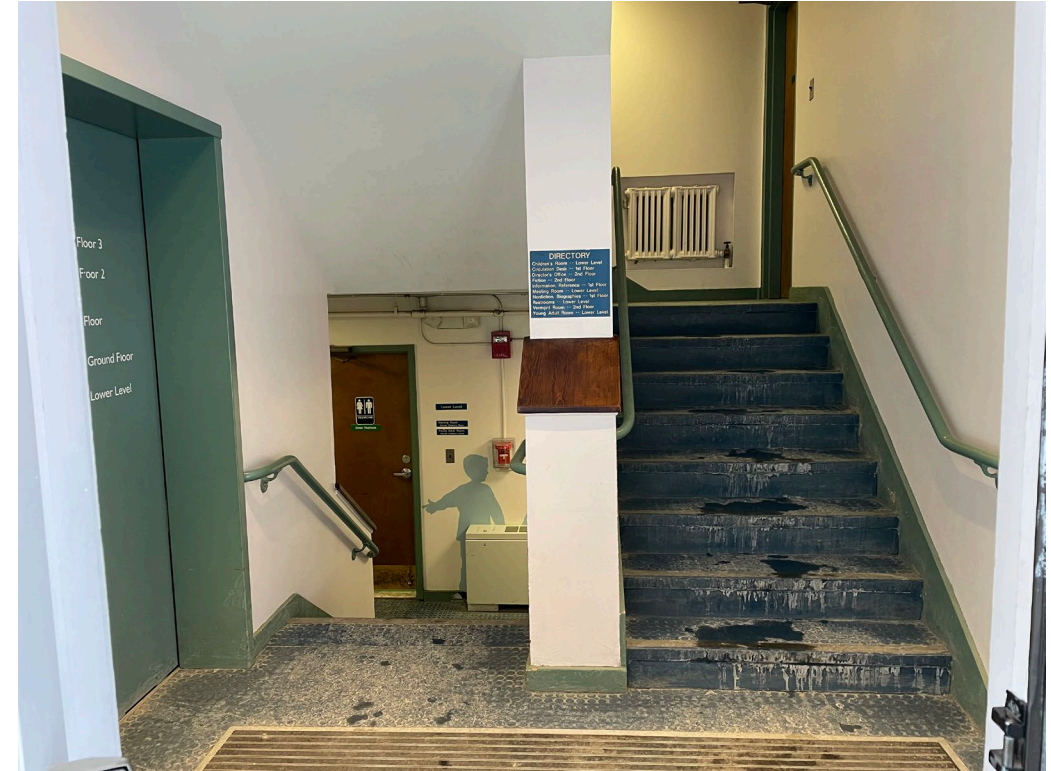
The library's primary entrance is not accessible; not welcoming; and provides unsupervised access to single occupancy restrooms.
