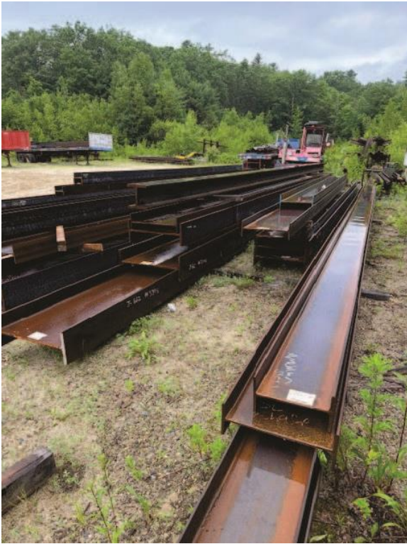
IPL Ph 1 steel structural elements, stored offsite, at American Steel Fabricators in Greenfield, NH
