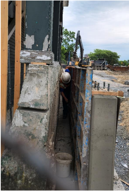
Tight quarters! An ECI employee must squeeze sideways between the south retaining wall of 71-73 Main and Ilsley's new northwest retaining wall, to strip concrete forms.
