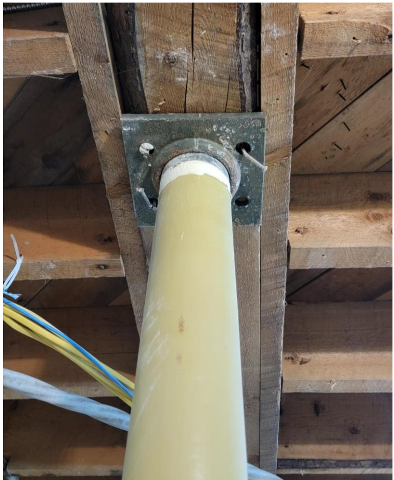
Basement: Peened over nails to be replaced by bolts
