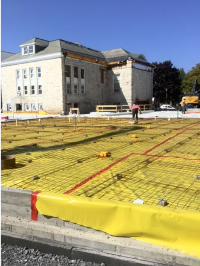
Ready for the last slab pour, pre-noon, September 15. Block chairs strategically placed, vapor barrier joints taped.
