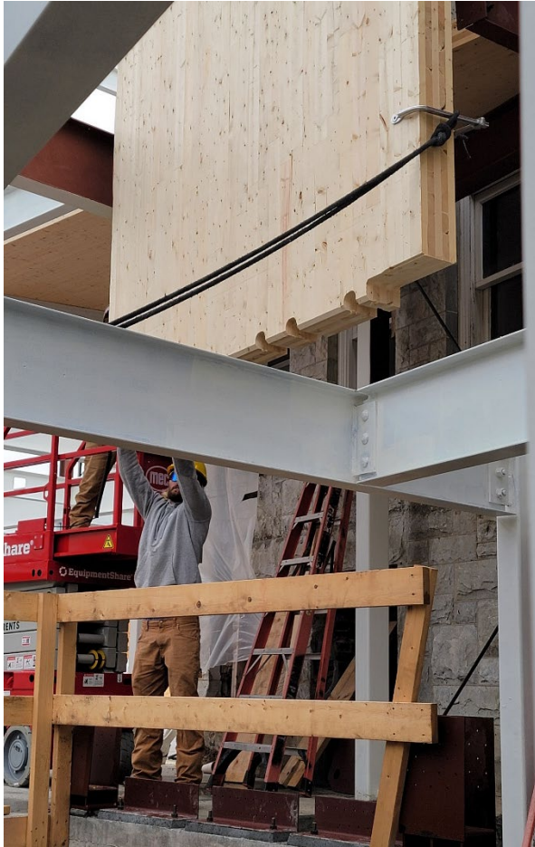
CLT can be used for walls, too! A 4,000 pound panel at elevator north wall dropping into place.
