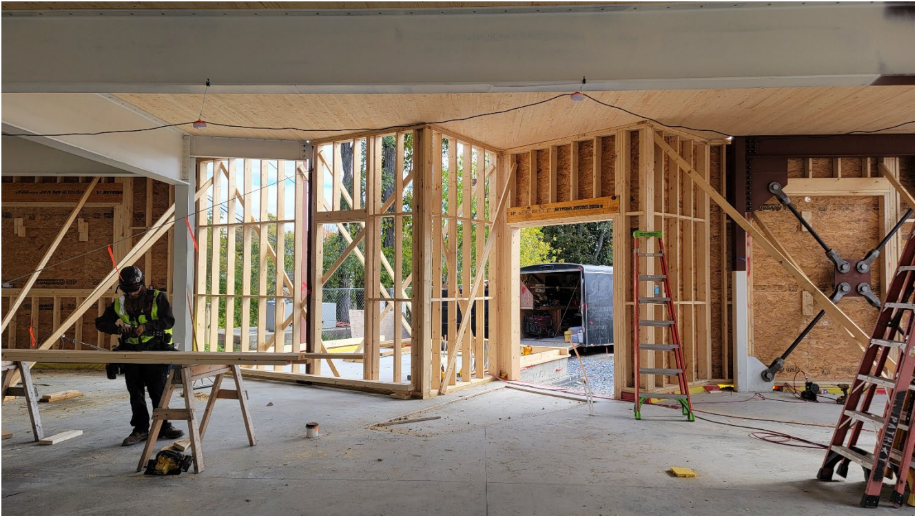
Patriot framing crews begin to pre-build exterior walls on the ground and install by standing them up to a surveyed reference line on the slab. New east public entrance off parking lot to Community Room (right) and door to Stair B shown (left).
