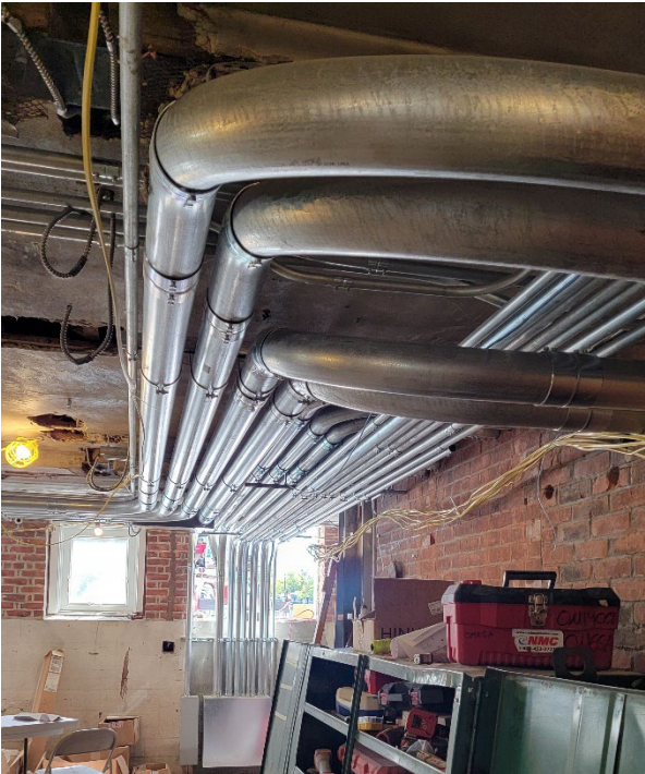
New electrical conduits snake through 1924 basement.
