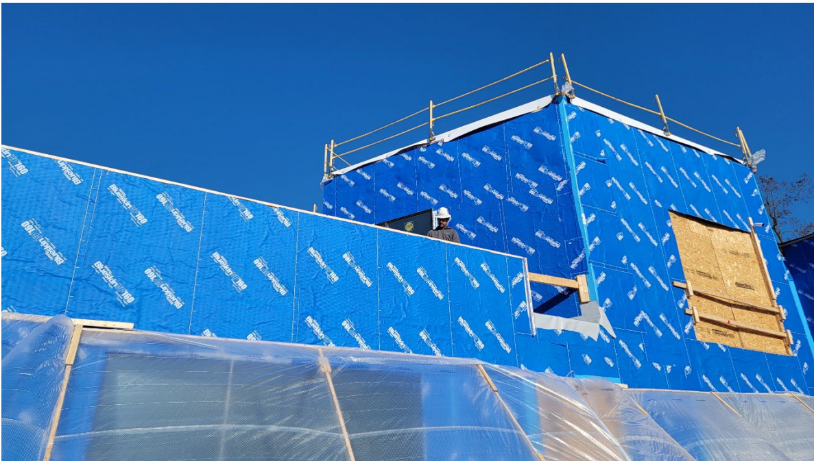
ROOF TERRACE parapet wall, reduced in height.
